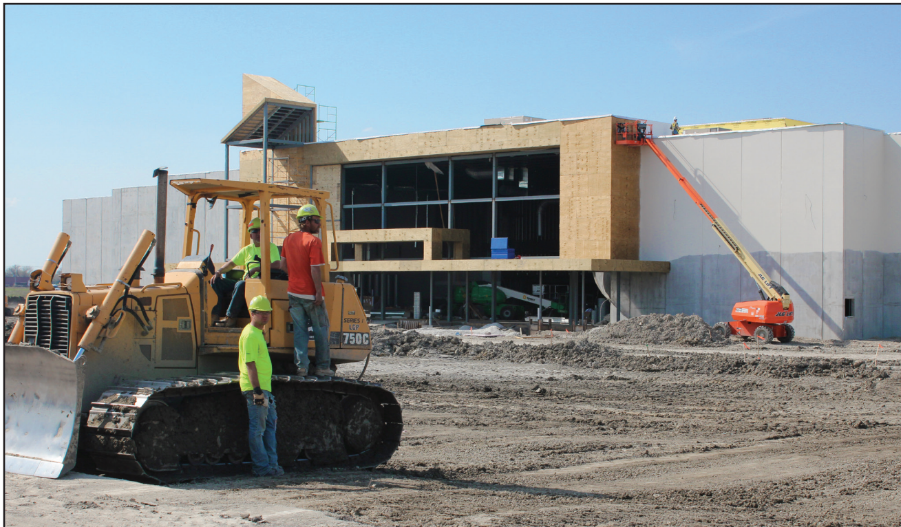
A construction crew works on renovations of the revamped Carmike 13 theater on April 30, 2013.
