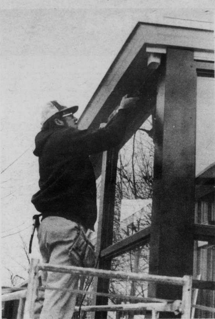
Finishing touches on the South Annex exterior continued up until time for the Open House. Photo by Ken Ferran
