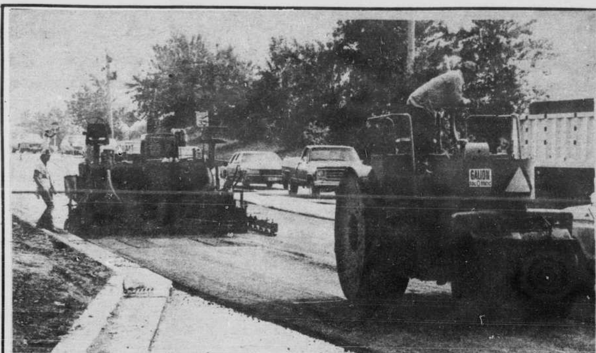
Traffic was backed up this past week as road crews put the finishing touches on the construction at Bradley and Mattis Avenues. Photo by Randy Pregler
