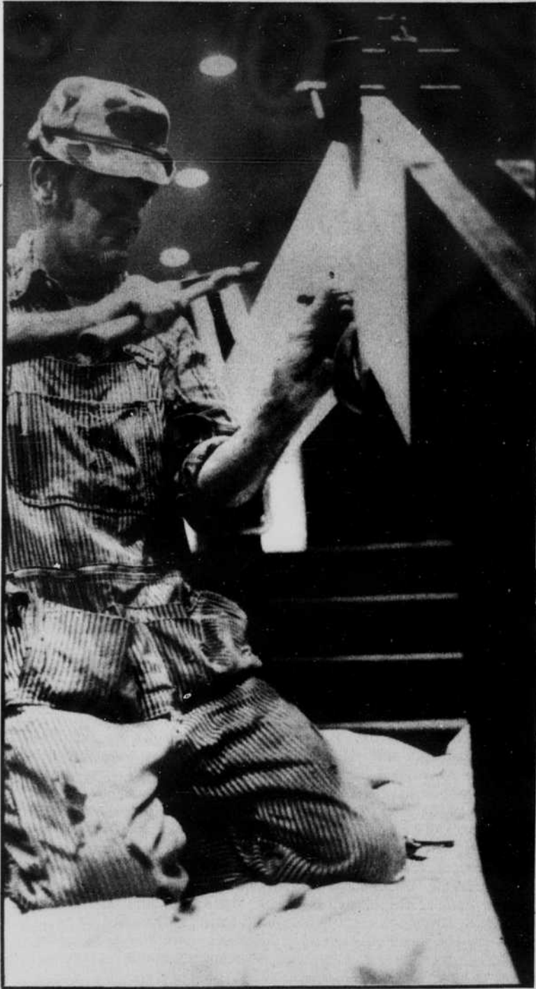
A workman repairs a hand rail in "X" section as the school re-vamps their handicapped facilities. The hand rails were extended to make things easier for blind students. Photo by Jerry Lower
