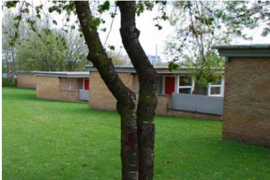
Figure 14. Photo of the single-family houses with flat roofs, poor thermal insulation in façades and gables, as well as many thermal bridges in the building envelope. From www.kildeparken2020.dk (with permission).
