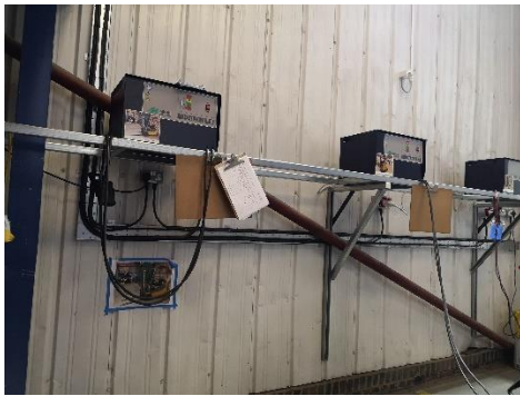
Photo 7 Forklift chargers on raised shelf
