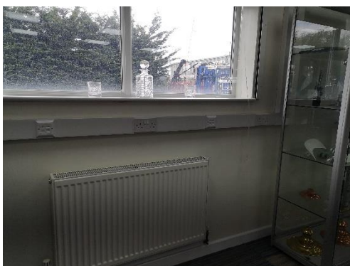
Photo 5 Raised electrical points
