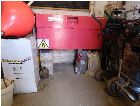
Photo 32 Petro tank on raised stand
