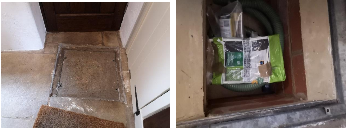
Photo 23/24 Electric water pump at the entrance
