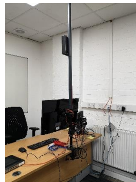
Photo 6 Cabling from the ceiling
