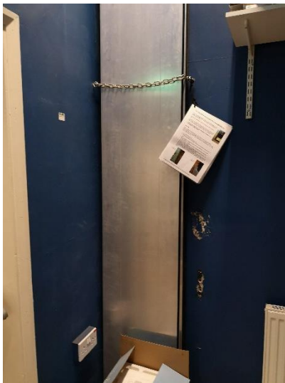
Photo 47 Flood gate boards with instruction
