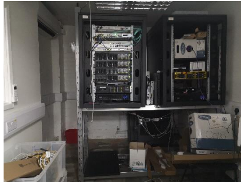
Photo 8 Servers on raised shelf
