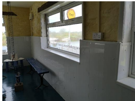
Photo 29 Raised electricity sockets
