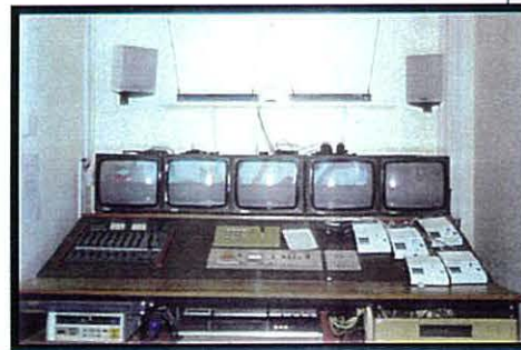
Video Control Room
