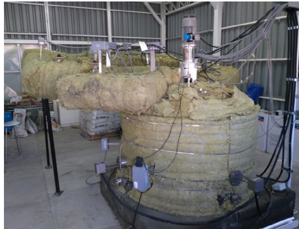
Fig. 4 Photo of pilot plant of molten salts of the University of Antofagasta.
