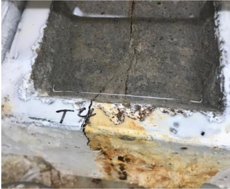
Figure 3.28: Cracking of the concrete in specimen Conv-B-3 during the cracked beam test
