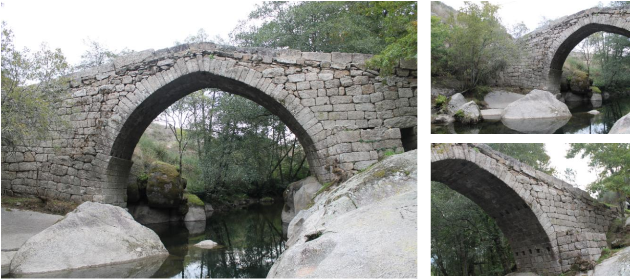
Fig. 3. 17 - Downstream side photos, Oct.16th 2015
