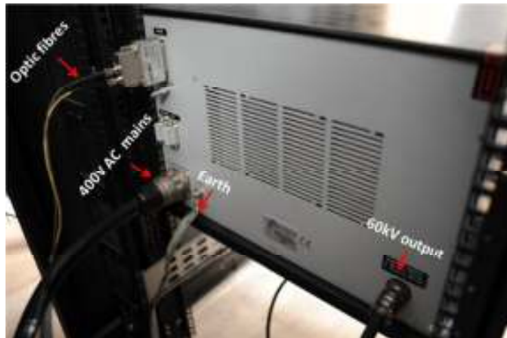
Fig 2.4: Rear view of D-bank Charger
