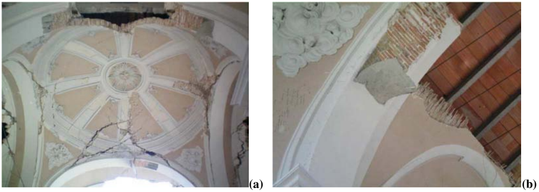
Figure A1.12 - dome collapse
