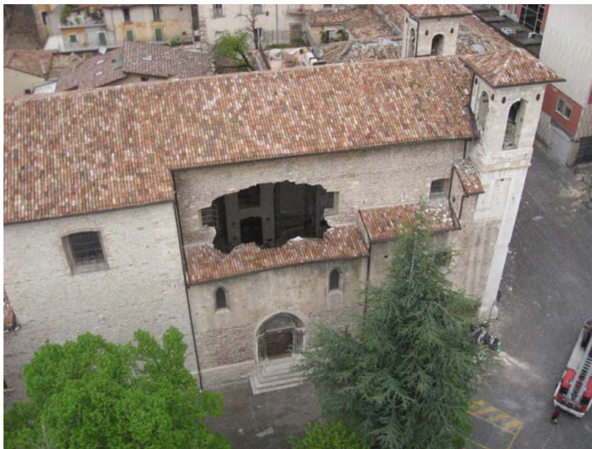
Figure A1.15 – left façade collapse
