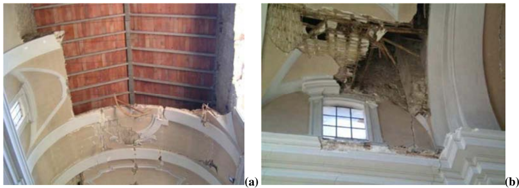
Figure A1.13 - barrel vault collapse
