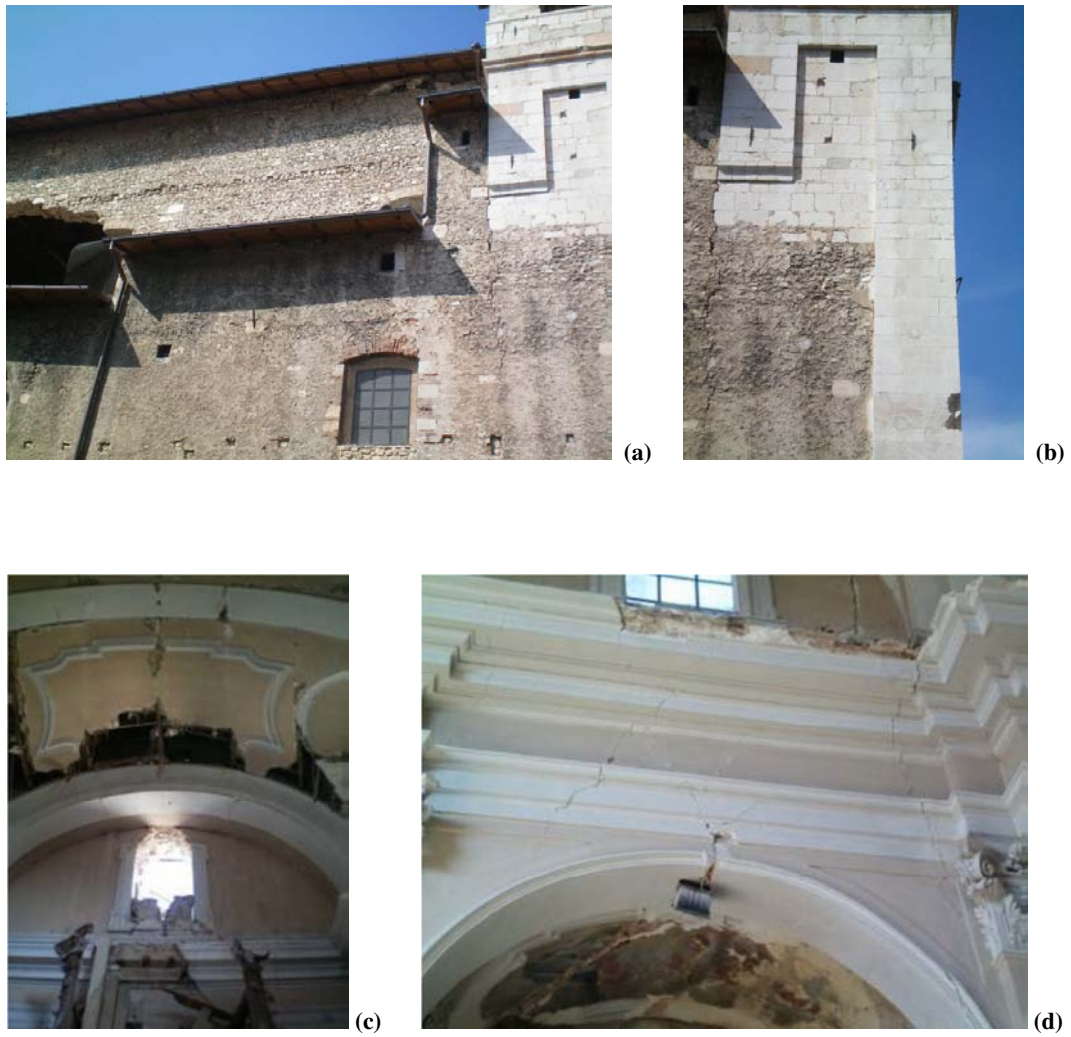
Figure 5.4 - Out-of-plane movement of the main façade.
