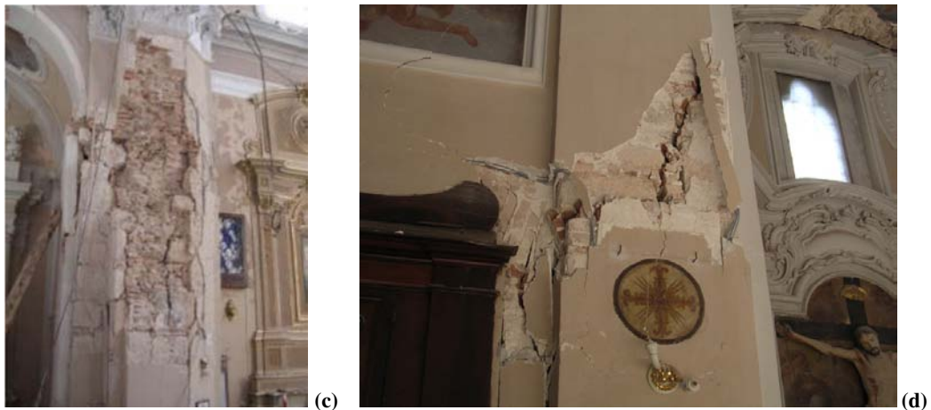
Figure 5.7 – Out-of-plane movement of the chapel walls.
