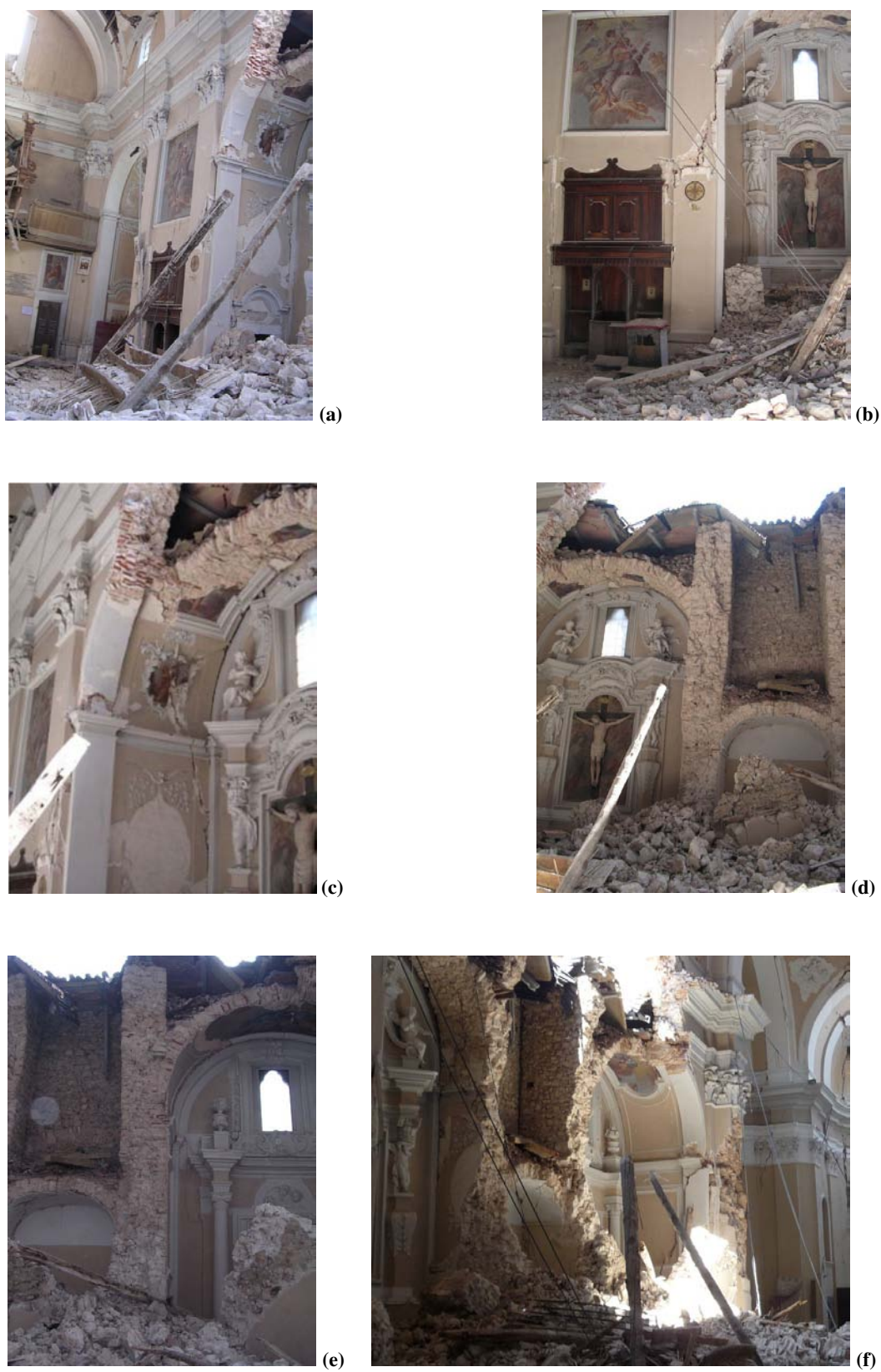
Figure 5.9 – Chapels vaults collapse.
