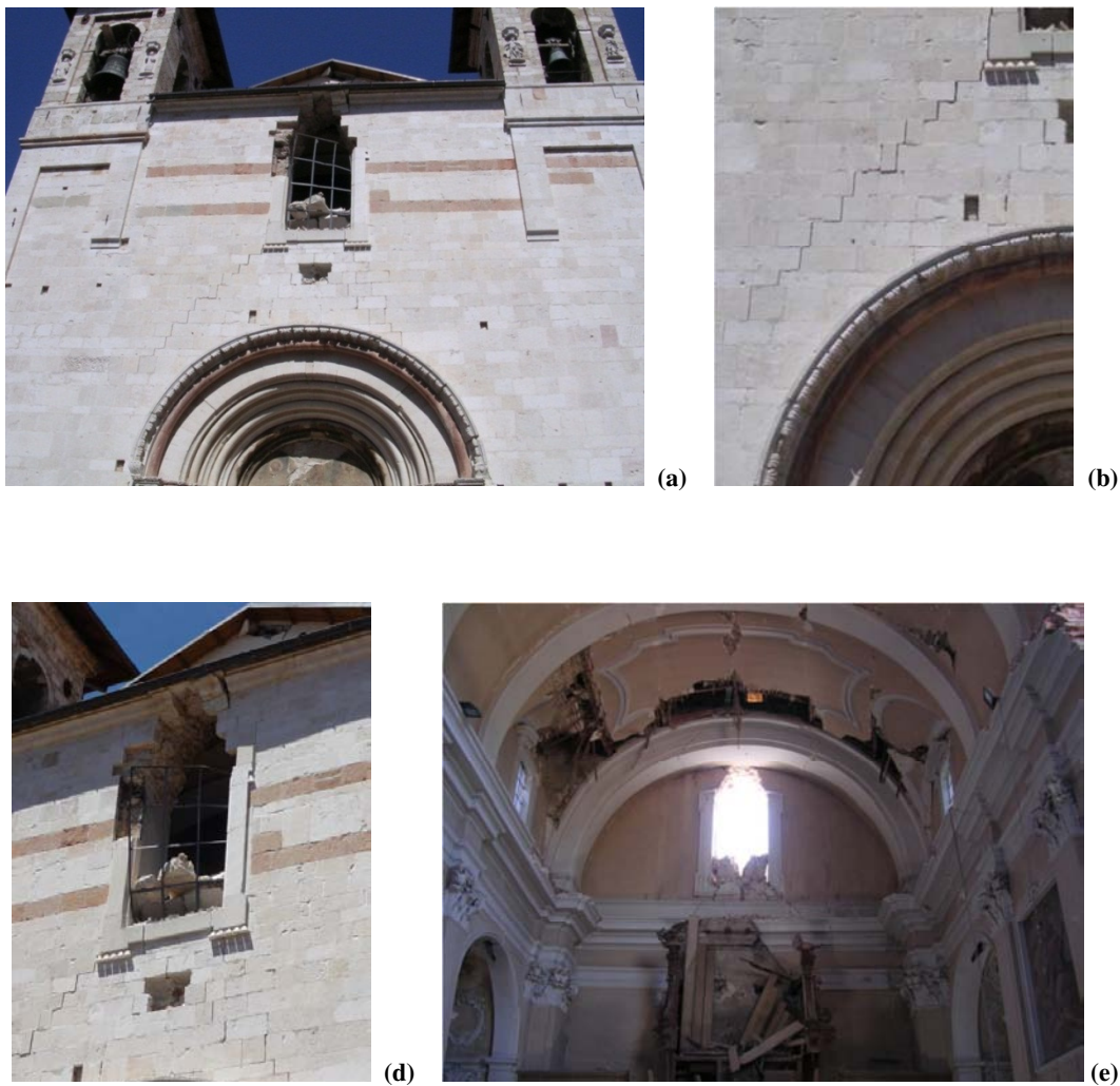
Figure 5.5 - In-plane movement of the main façade.
