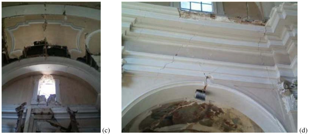
Figure A1.16 - Out-of-plane movement of the main façade.
