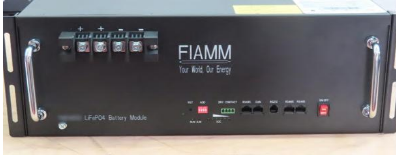
Figure 4.41: Battery Pack n.3
