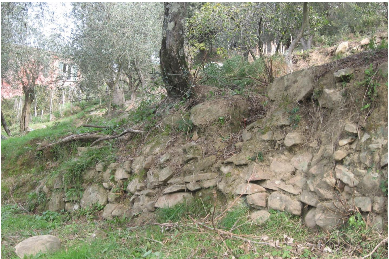
Figure 4.3. Partial terrace wall failure.
