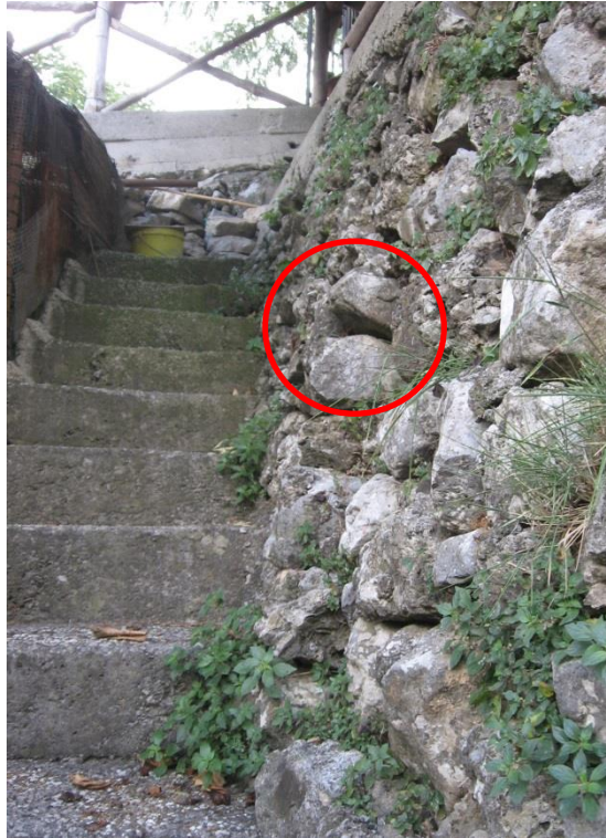
Figure 4.11. Bulging in the wall middle part in Tramonti.
