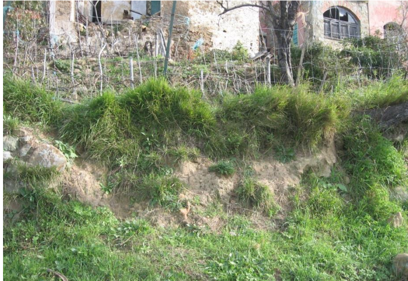
Figure 4.2. Collapsed section of a terrace wall.
