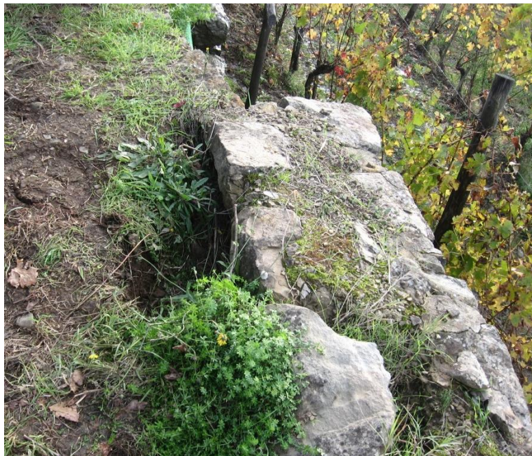
Figure 4.7. A new wall seen from the top. It can be noted that because of the bulging the wall has slightly shifted onwards.
