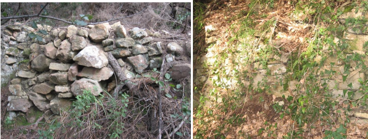
Figure 4.1. Bulging and partial degradation in terrace walls in Case Lovara .
