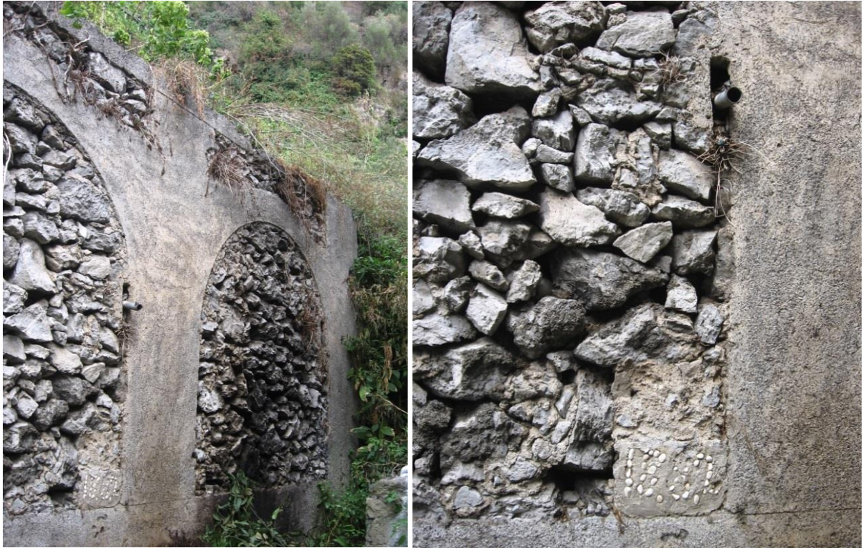
Figure 3.21. a) Terrace wall with supporting arches in Maiori; b) at the basis of the wall the year of construction can be read: 1887.
