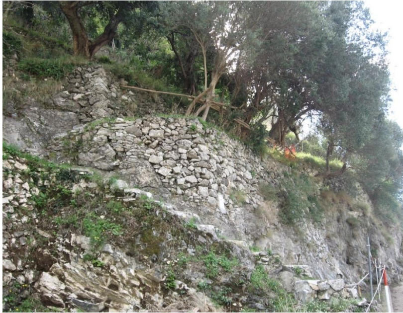
Figure 4.14. Terraces cultivated with olive groves in Minori. Terrace walls show a poor building technique respect to walls supporting citrus groves.
