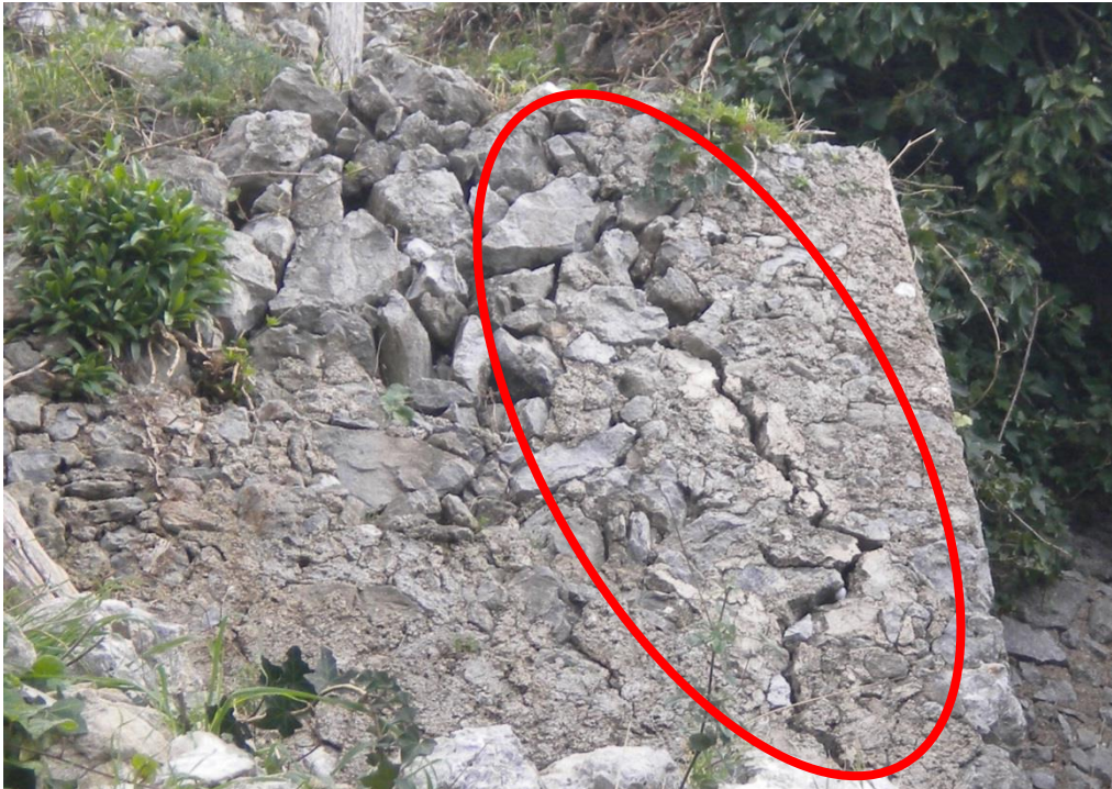
Figure 4.1222. Crack in a wall pillar in Maiori.
