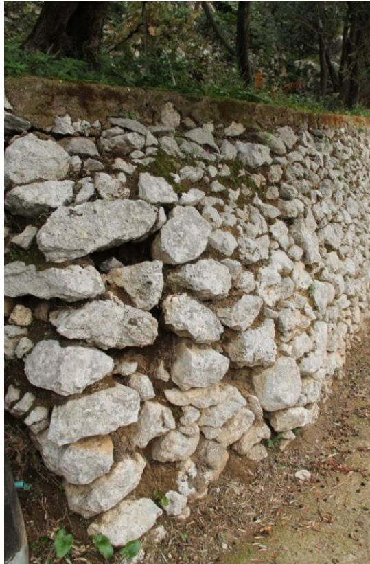
Figure 233. Gaps in the wall in Ravello.
