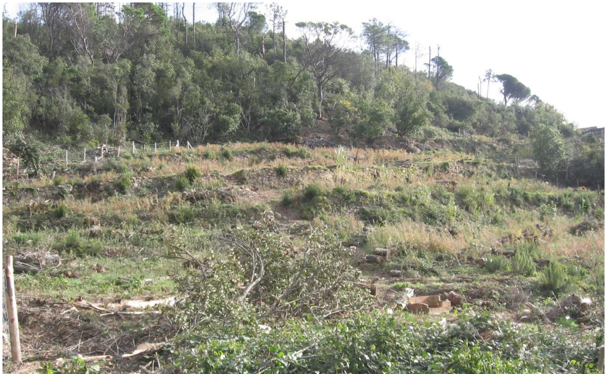
Figure 3.5. Another section of the property. Even if terraces have been cleared by the most of the invasive vegetation, most of the walls are seriously damaged and without traces of old cultivations.
