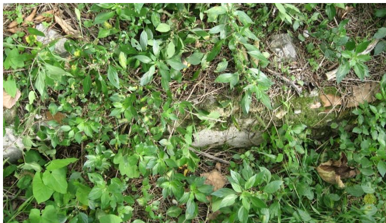
Figure 4.18. Pipeline in mortar full of vegetal debris and invasive vegetation in Maiori.
