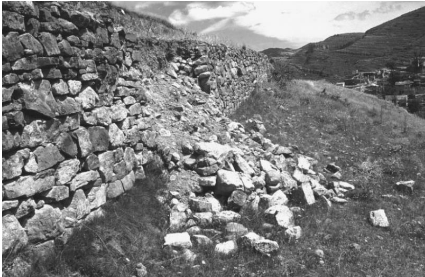
Figure 2.6. Collapse of a terrace wall at the foot of a hill near a village, resulting from hydrological pressure higher up (Leza Valley, La Rioja, northern Spain). Fields in this gently sloping area were only abandoned within the last 10 years (picture from Lasanta et al., 2001).
