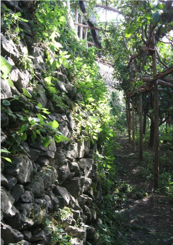
Figure 4.10. Bulging in the wall middle part in a cultivated terrace in Minori.
