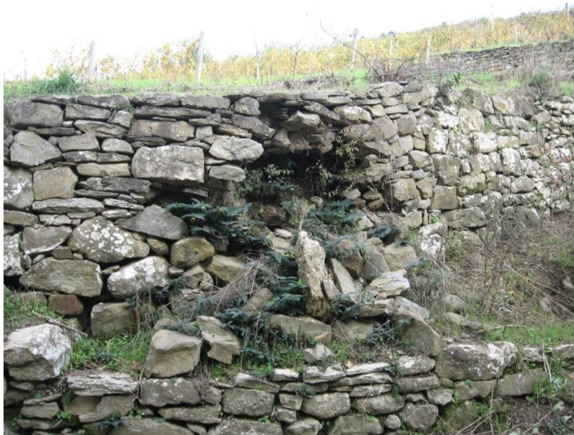
Figure 4.5. Collapse in an old manufacture wall.
