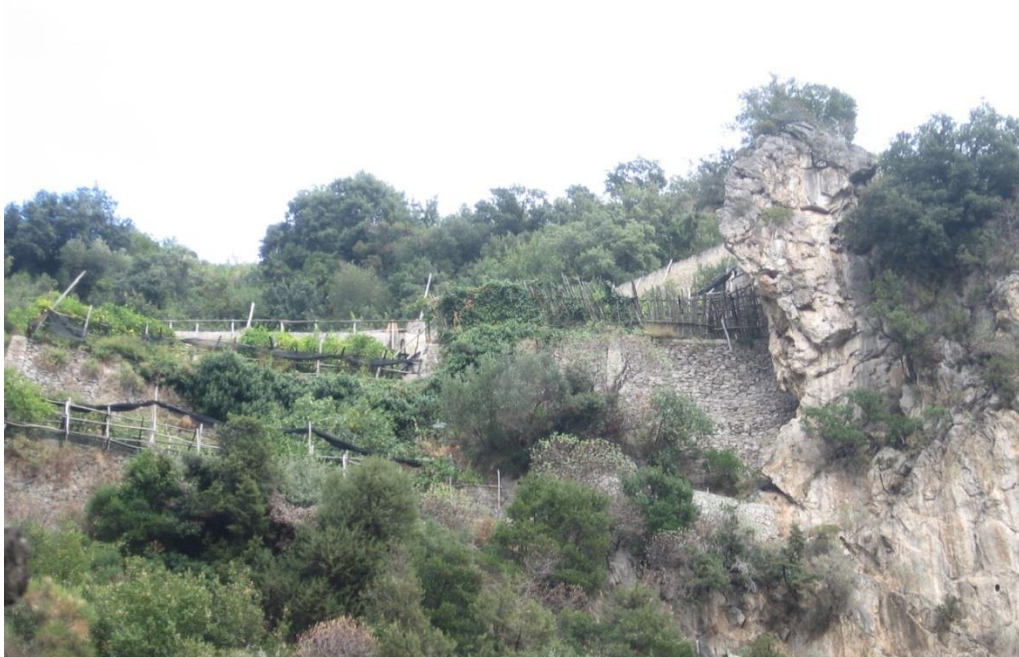
Figure 20.16. Spectacular terrace wall almost 10 m high built on a vertical rock cliff in Maiori.
