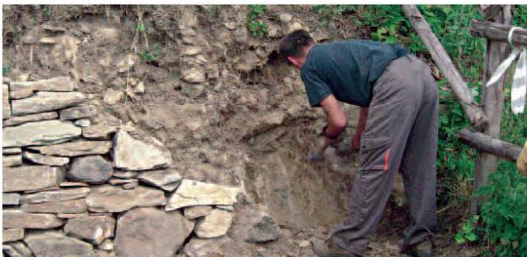
Figure 5.14. Remaining part of the wall in the form of a ladder to prepare the junction (picture from Sangiorgi et al., 2006)
