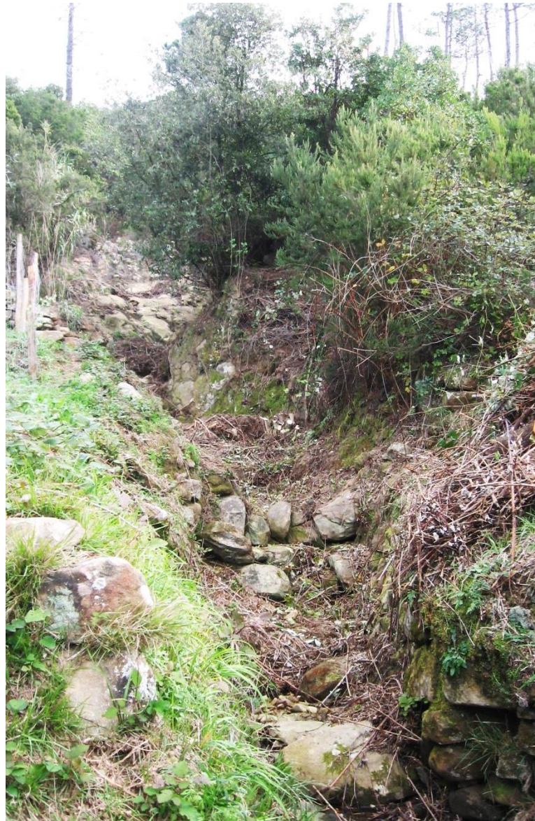
Figure 4.4. Drainage collection channel, abandoned and obstructed by invasive vegetation (now partially removed) and debris.
