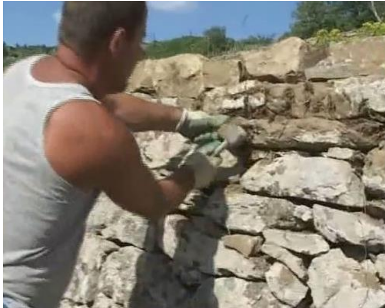
Figure 5.16. Stone settling during a dry wall construction in Lamole (picture from http://www.fattoriadilamole.it/ ).
