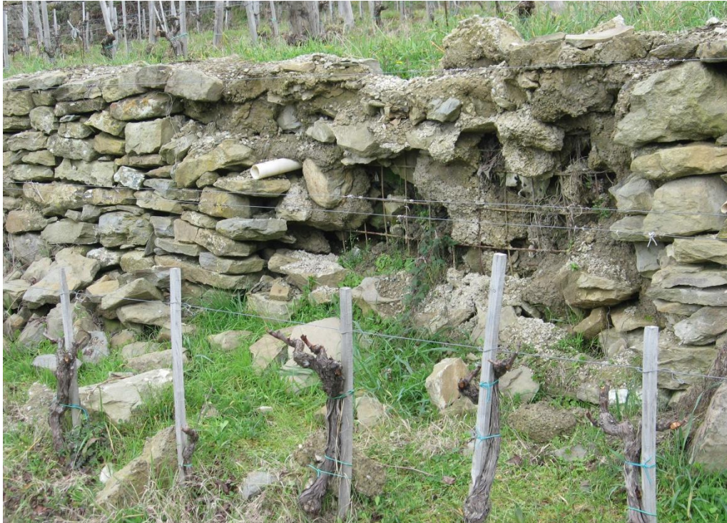
Figure 4.8. A new manufacture wall, already fallen. Drainage plastic pipes can be seen (picture by S. Calligaro).
