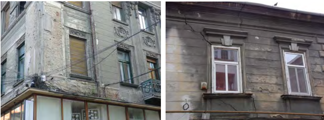
Fig. 1.8.8: Non-structural and structural damage (US 133 and US 71)
