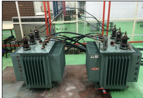
Figure 1. Photo of a distribution transformer with a capacity of 100 kVA
