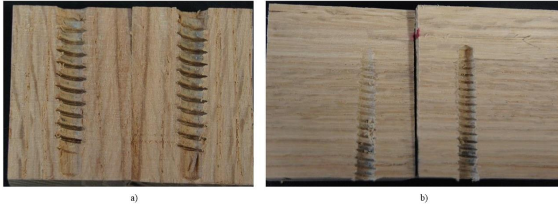
Figure 2.14 Cut views of a) #301 (C1) connection specimen's rail member and b) #302 (C2) connection specimen's post member, where a lag screw and hanger bolt were driven, respectively
