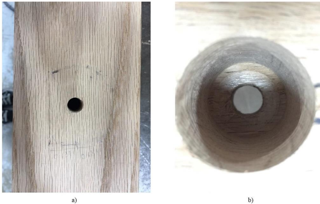
Figure 2.12 Perpendicular-to-grain compression failure examples for #301 (C1) post members in contact with a) rail members and b) lag screw washers
