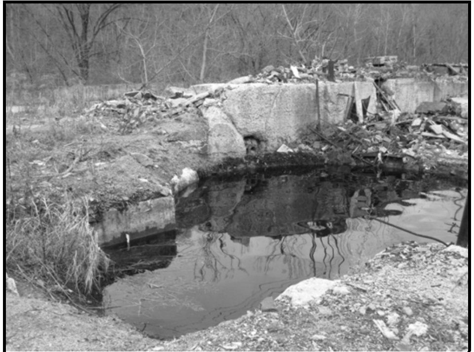
A pit full of dirty water creates a physical hazard at the Clinch River Corporation Site in Harriman, Roane County.
