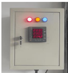
Fig. 16. Power Meter Panel Installation Results
