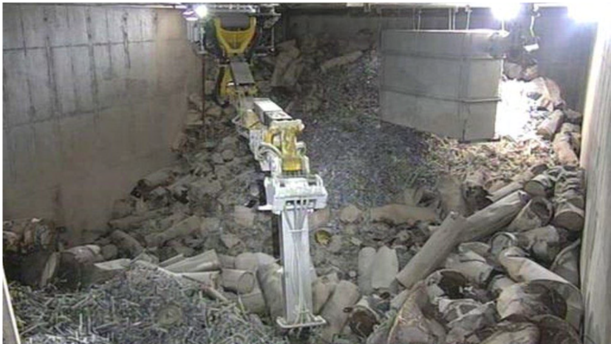
Figure 1.4: A photograph of the retrieval operation inside the Berkeley vaults [67]. A wide variety of wastes can be seen, including pipework, PPE and construction rubble.
