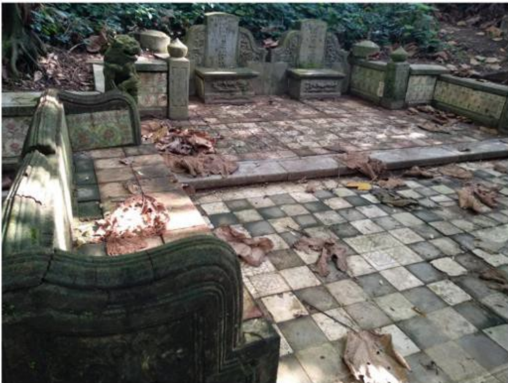
Figure 15: After the clean-up of the double grave, the benches and grave architecture can be clearly seen. Photograph taken in August 2020.
