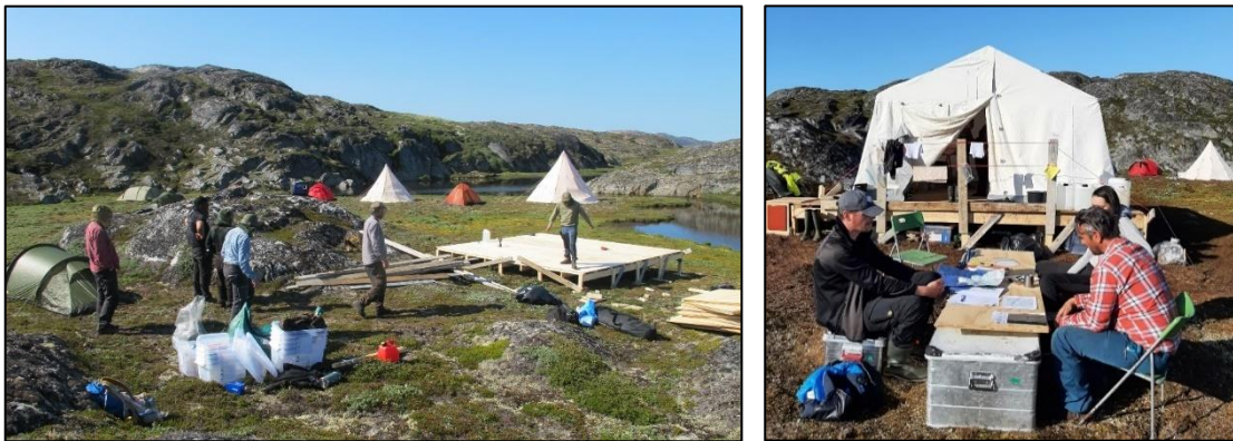
Left: Construction of plywood floor for dining tent at Nipisat. Right: Dining tent at base camp on Nipisat. (Photos: Jens Fog Jensen).
