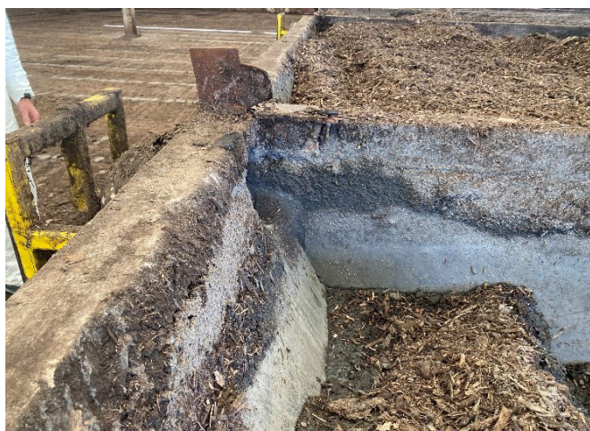
Figure 4. Front-end of the composting pit row, showing the manure inlet and space created for manure addition after the mixing vessel has passed through the fresh compost feedstock.
