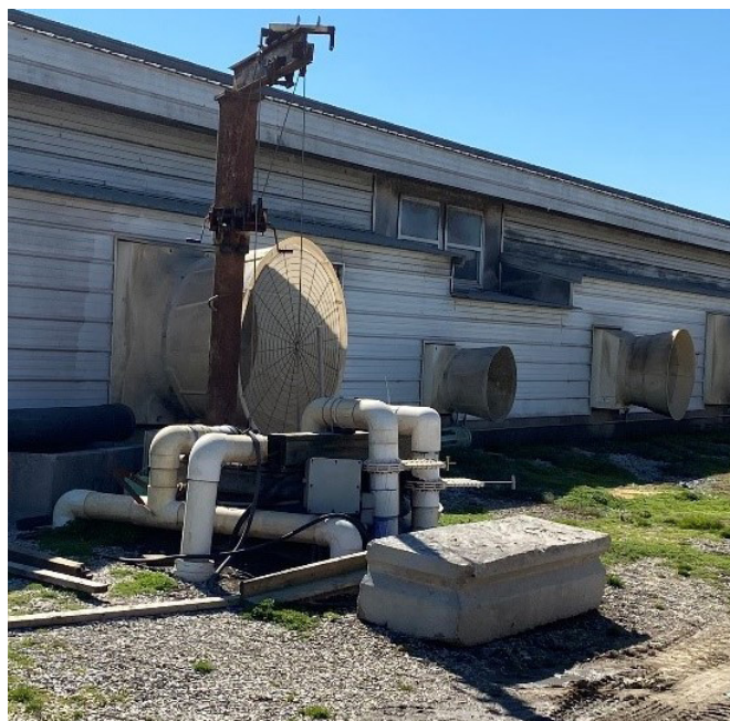
Figure 3. Lift station for pumping recently scraped manure from the finishing barns to the composting facility.
