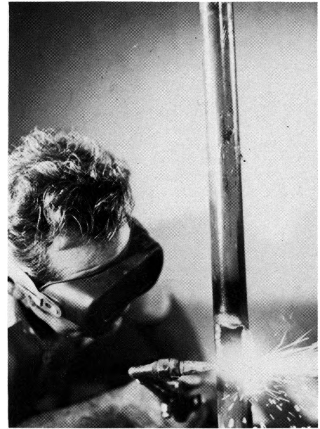
Larry Clark welds a pipe while working on the engineering renovation. Read Linda Kral's story on page 6. Picture by George Higginson.
