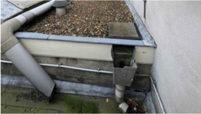
5 Down pipe system | urgent improvement needed
