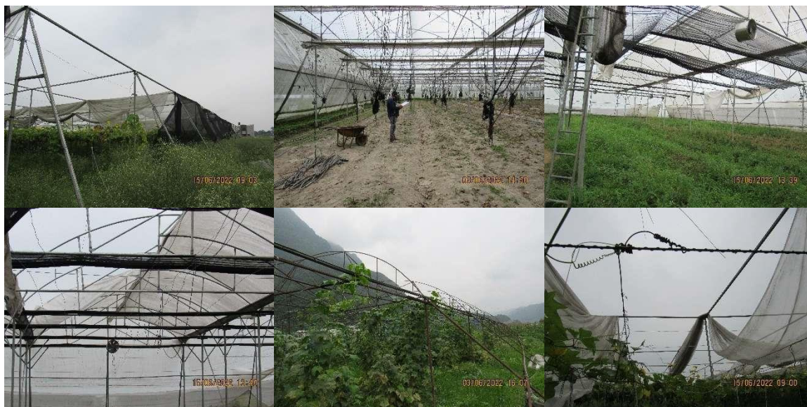
Figure 7. Poor management and damaged protected structures constructed with high investment in addition to government subsidy
