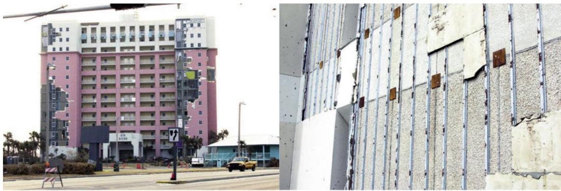
Figure 8. Detachment of the plasterboard panel from the wall substructure in Pensacola (Florida) [34].
