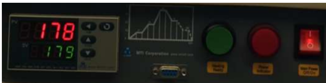
Figure 7: Small Programmable Tube Furnace Control Panel
