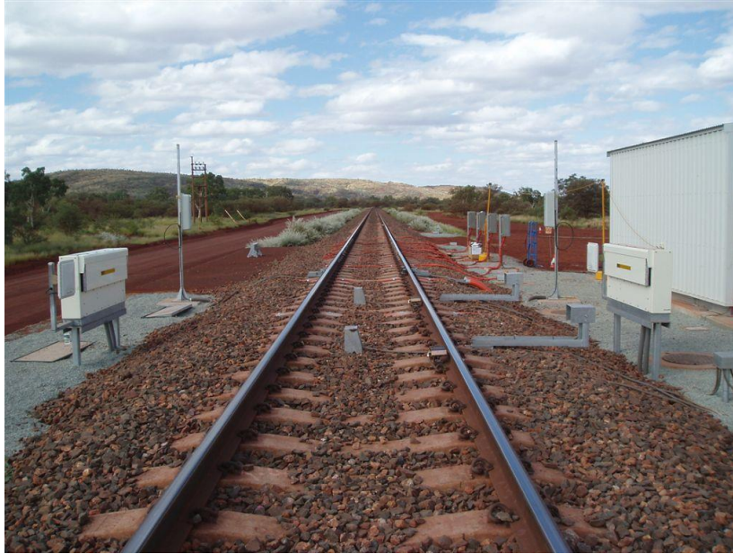
Figure 4. On-site RailBAM® system [9]
