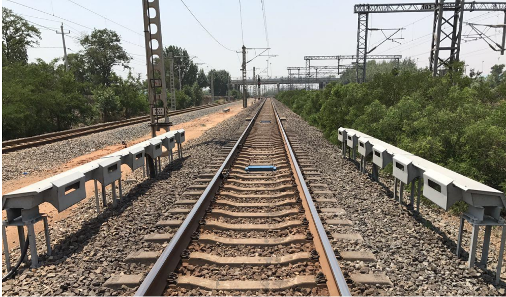
Figure 3. On-site Trackside Acoustic Detection System [6]
