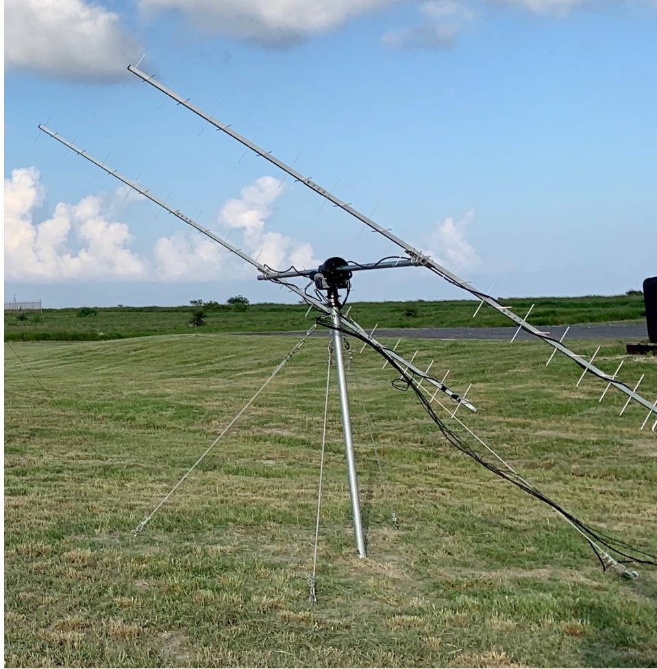
Figure 3.2: A completed antenna assembly installed outside the UTRGV STARGATE facility.
