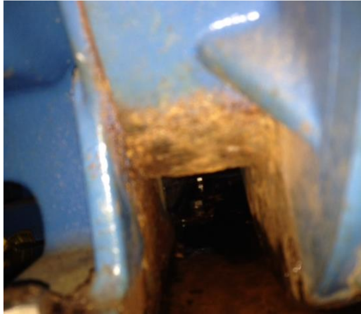
Figure 3. Left-side view of rust around the leak-hole.
