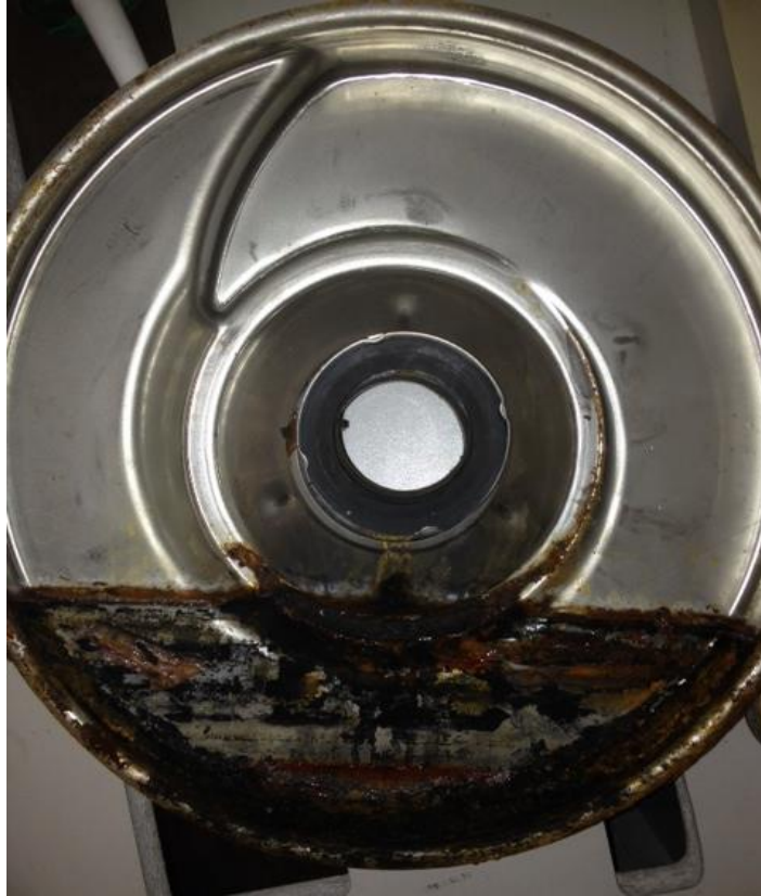
Figure 5. Rust on the interior side of the casing
