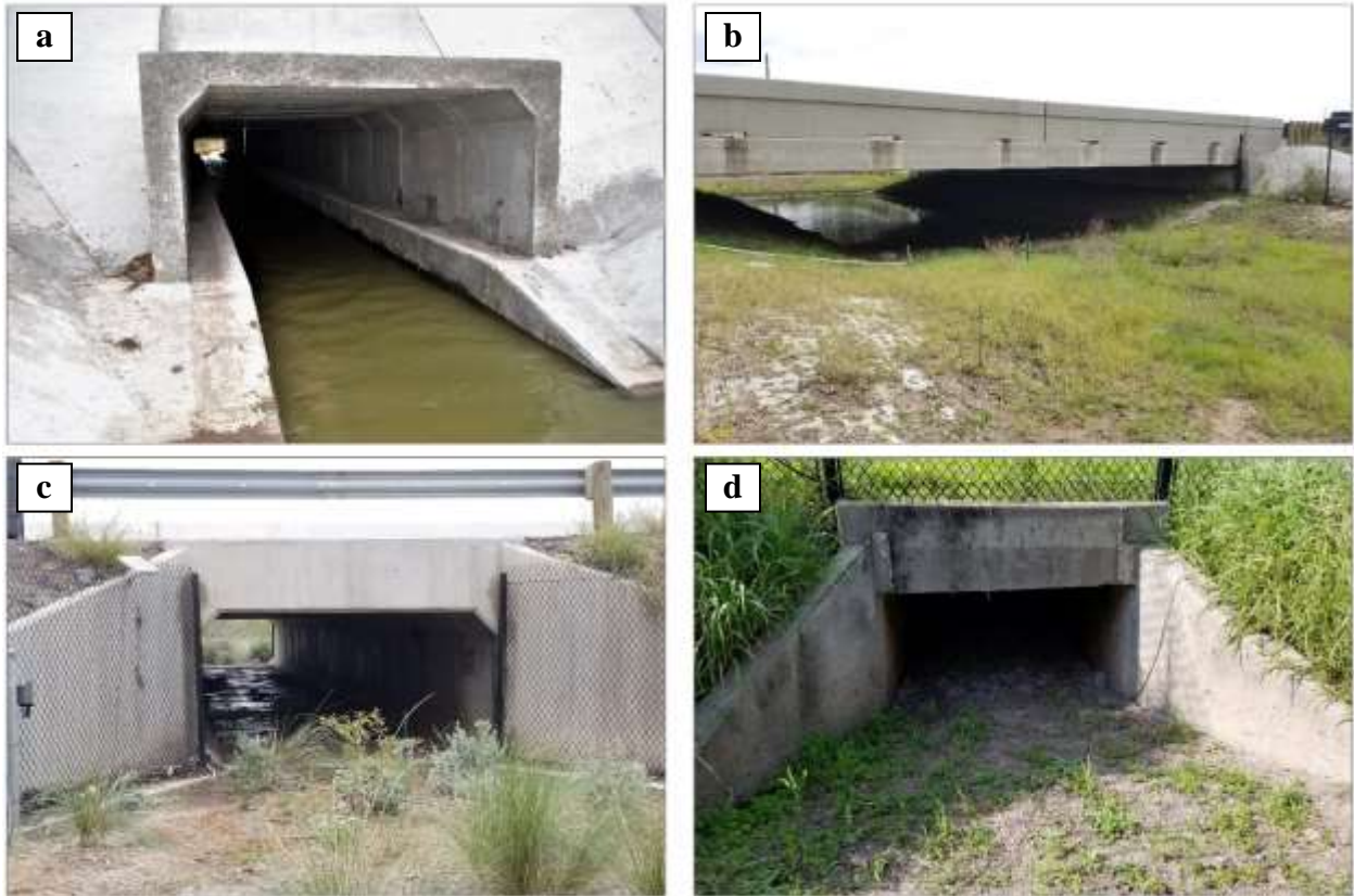
Figure 2. Four of the five wildlife crossing structures (WCS) constructed by the Texas Department of Transportation to address ocelot ( Leopardus pardalis albescens ) mortality along State Highway 100 in Cameron County, Texas, USA. From top left: WCS2 (a), WCS3 (b), WCS4 (c), and WC3A (d). WCS1 is not pictured because it has the same configuration as WCS2.
