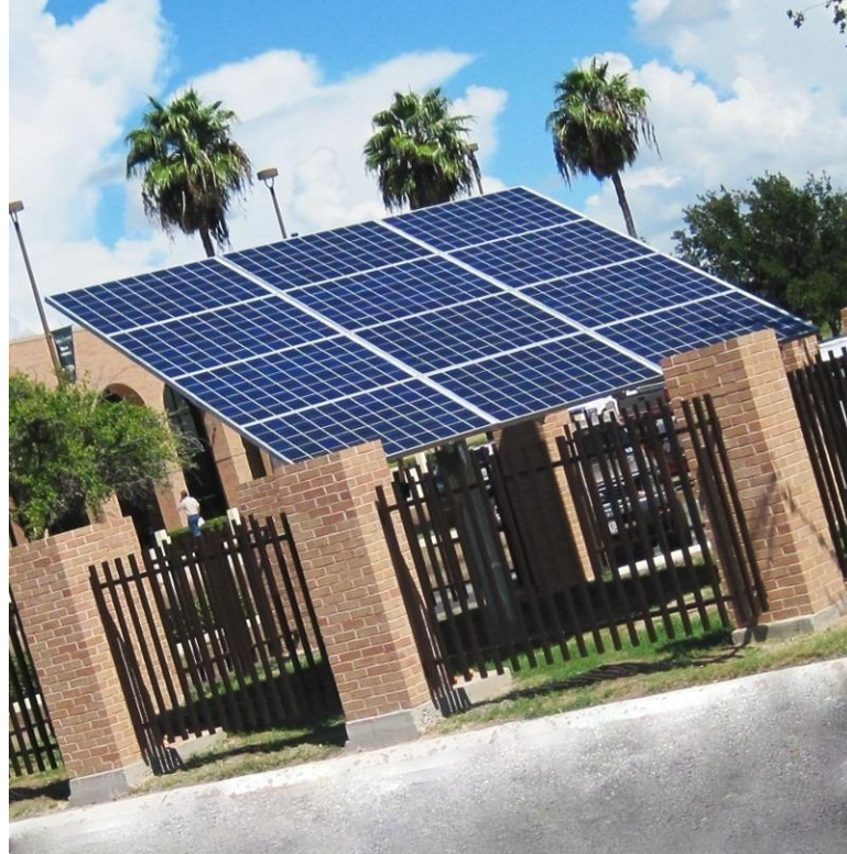
Figure 3.2 - North Half of the TXU Sun Tracking Arrays at UTPA
