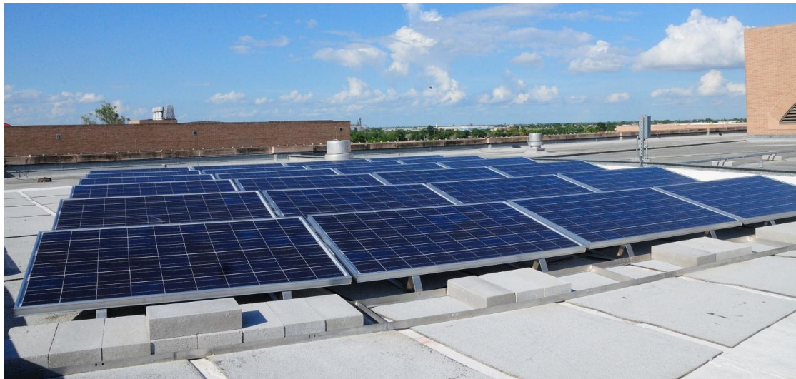
Figure 3.1 - ENGR PV Array at UTPA Engineering Building rooftop
