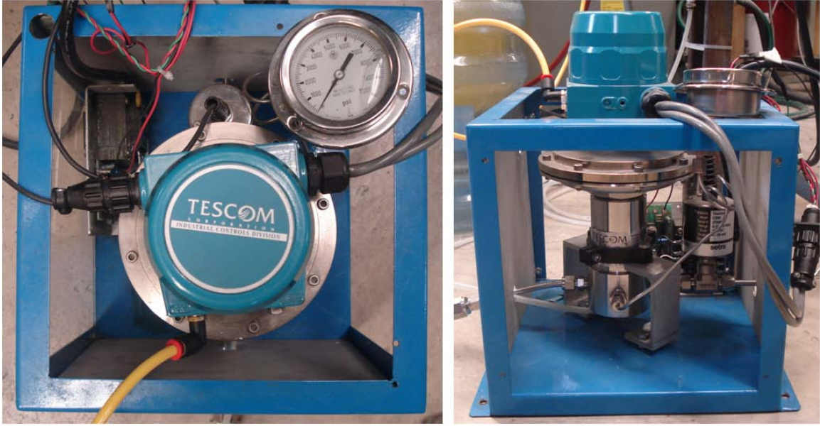
Figure 10. Gas pressure regulation control unit.
