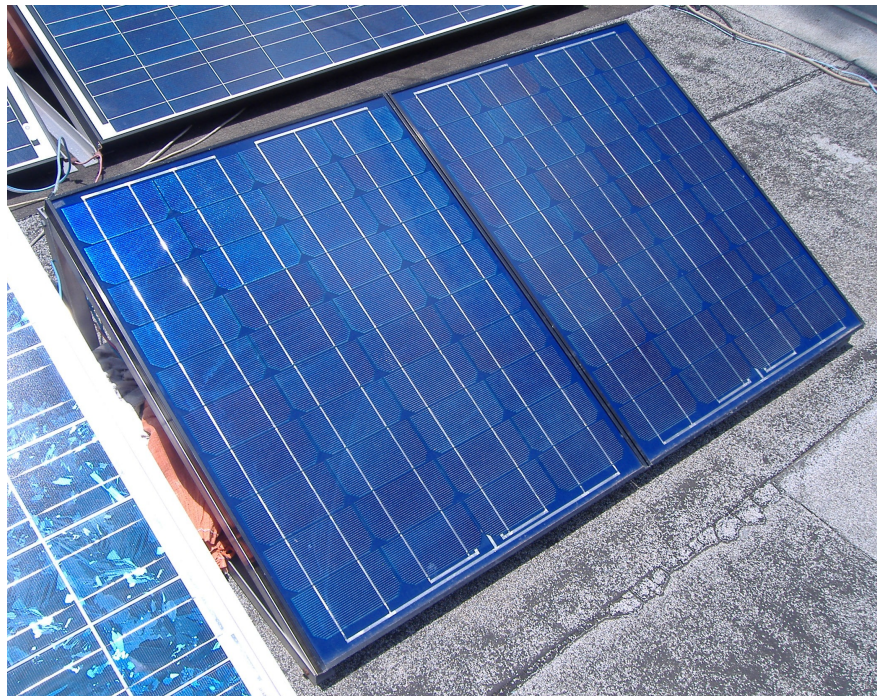
Figure 10: General Electric 50 W PV Solar Panels (Qty. 2)
