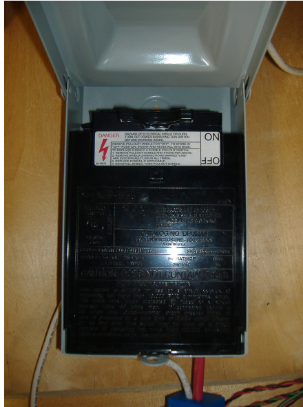
Figure 12: Safety Cut-off Switch
