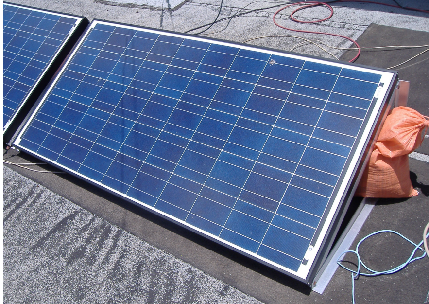
Figure 9: BP 200 W PV Solar Panels
