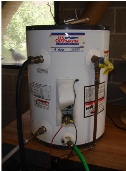
Figure 19: Water Heater With Heating Coil
