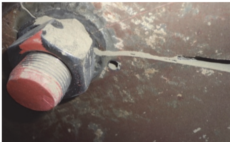
Figure 4: Crack that propagates towards the bolt hole.
