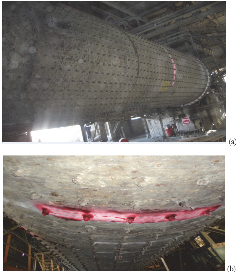
Figure 6: Crack repaired (a) far or perspective view of the crack, and (b) near view of the crack
