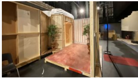
Making sure that each of the seven doors onstage has its own reveal wall – a setting that shows what lies behind the door – was a challenge for scenic designer Mandy Goynes while building the set for the Ole Miss Theatre production of 'Boeing, Boeing.' Photo by Katherine Stewart/Department of Theatre and Film
