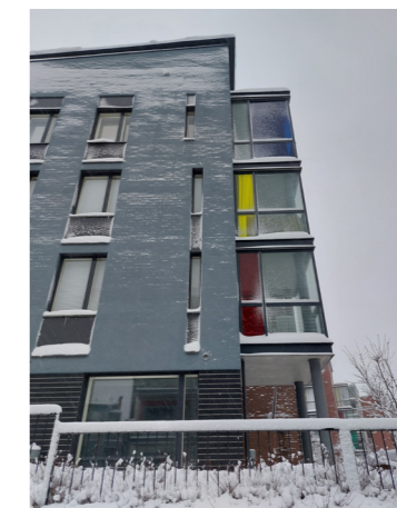
Figure 3.3.3.1 Snow attached to the façade, January 2022, Uusimaa
