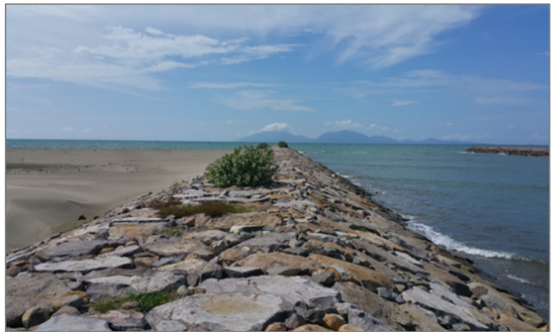
Figure 7. Condition of jetty at point 6
