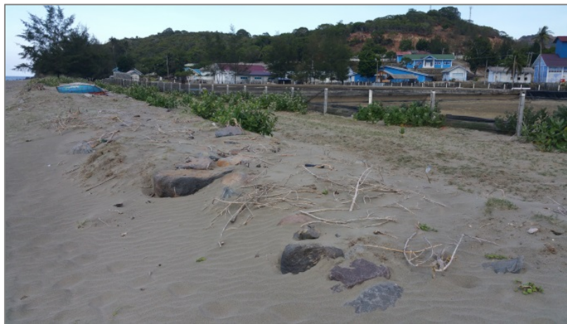
Figure 11. Condition of jetty at point 9
