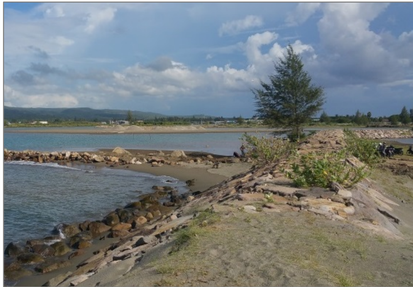
Figure 8. Condition of jetty at point 7
