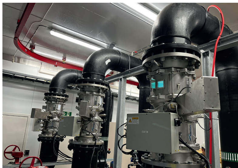
Atlantium RZB300 HOD installation for sea-water IPN protection. Photo: © Atlantium
