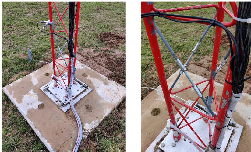
FIGURE 2 Photograph of the foundation and anchor plate (left), and photograph of the first bay and damage mechanism in place (right)
