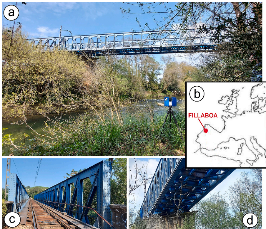
Fig. 20. Railway bridge over the Tea River a) Front view of the first span of the bridge b) Map of the bridge site c) View of the interior of the bridge d) Bottom view of the structure.
