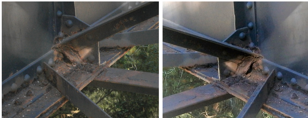
Fig. 9. Details of the corrosion state in two of the girder-bracings connections.
