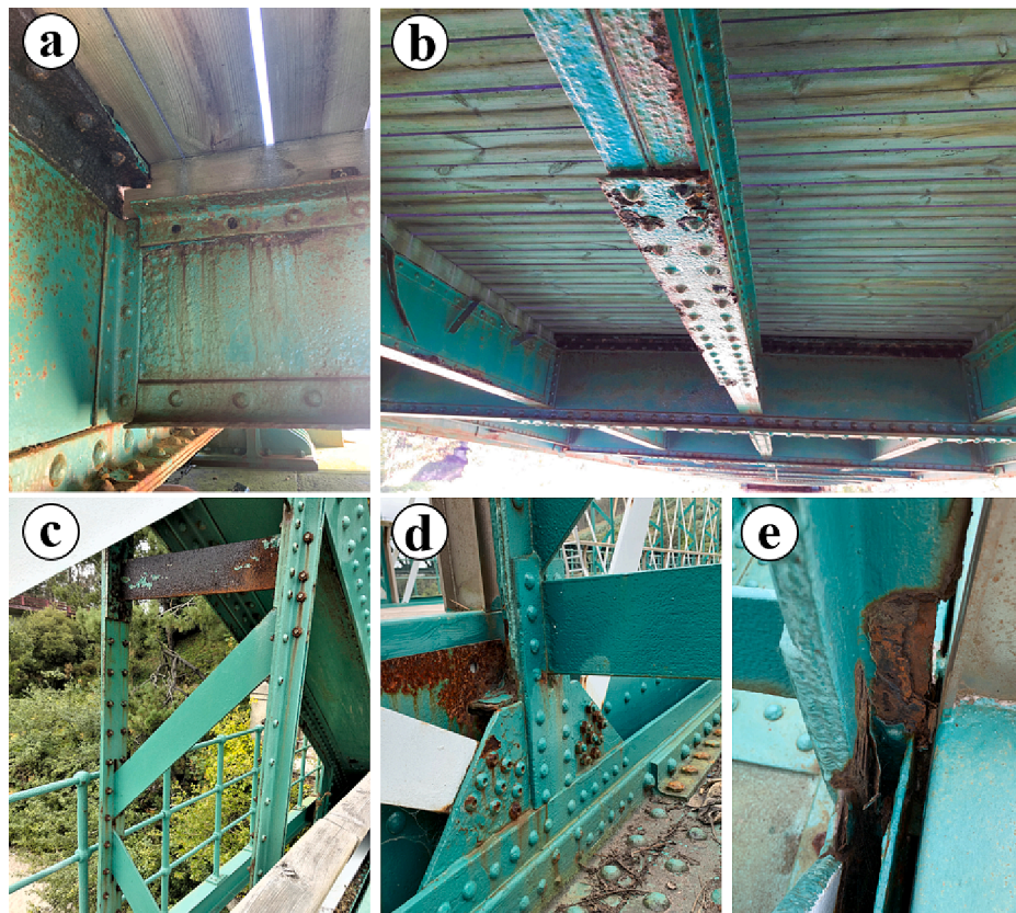
Fig. 5. Examples of damaged and retrofitted elements in O Barqueiro bridge: a) Lack of rivets in a stringer b) detachment of the flange plates c) rivets replaced by bolts d) retrofitted hanger e) corrosion in the lower part of a hanger.
