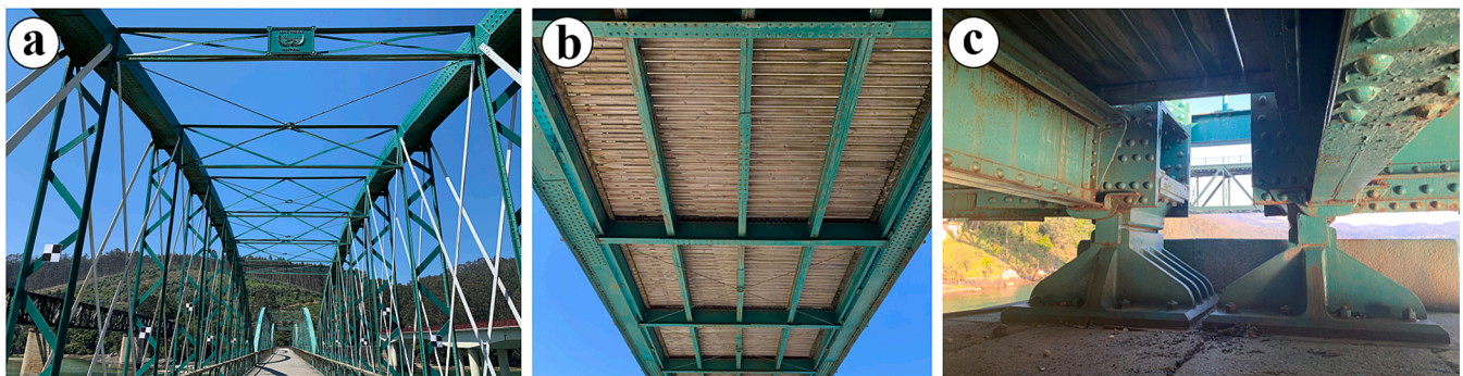
Fig. 3. Details of O Barqueiro bridge: a) arch ribs, vertical hangers, sway systems, and cross bracings b) tie girders, cross-girders, and stringers c) supports.
