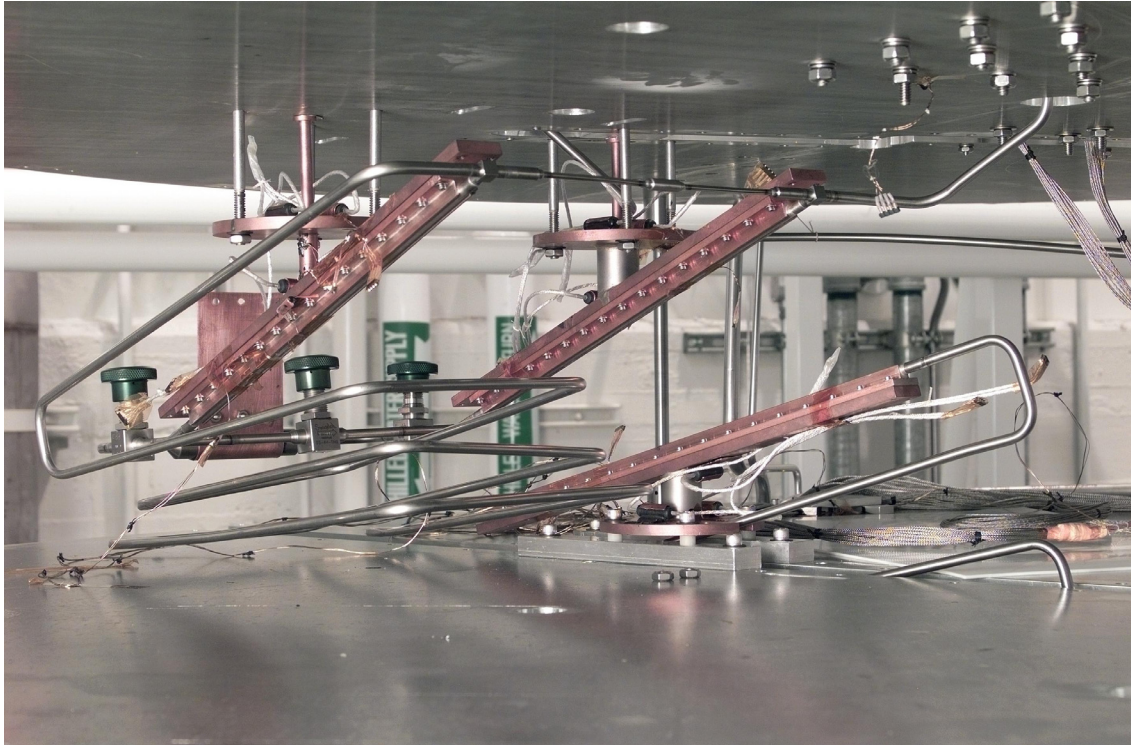
Figure C. Photograph of 100K and 55K pre-coolers (PC2, PC3a, PC3b)
