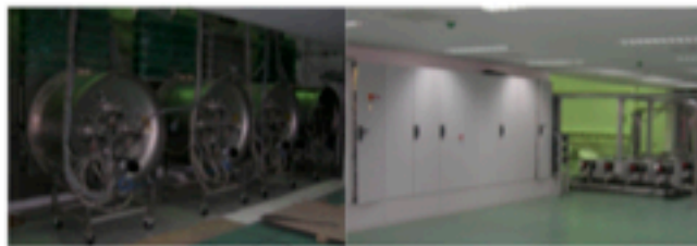
Figure 1-6: Example of cryogenic vacuum system complete of helium compressors and electrical cabinets (for reference only)
