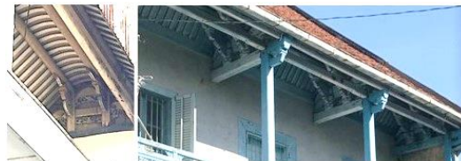
Fig. 17: Purlin supporting by roof console of the Chinatown in Semarang Source: Sudarwani et.al, 2022
