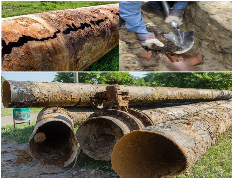
Figure 1-2: Different Pipe Deficiencies.
