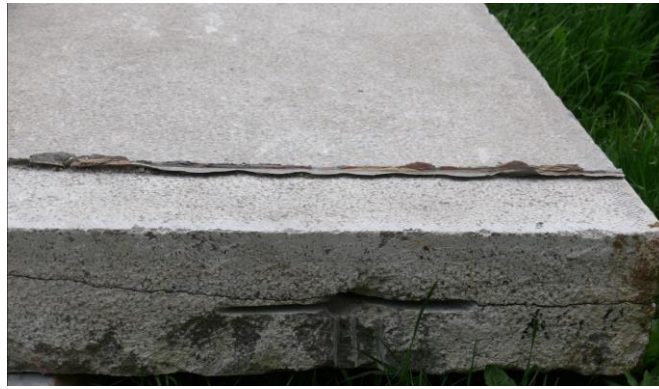
Figure 6-2: Delamination of concrete deck slab.
