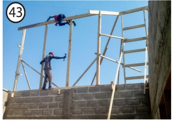
Picture # 43: Erecting roof trusses without any forms of fall arrest systems
