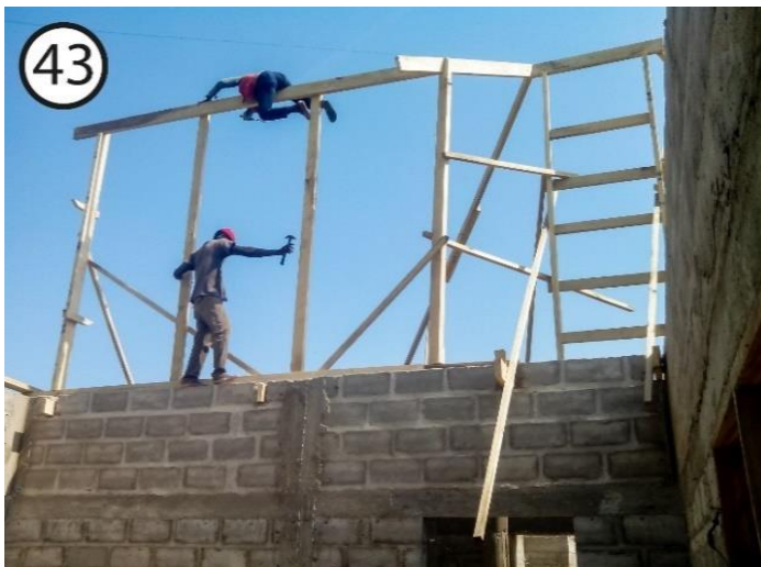
Picture # 43: Erecting roof trusses without fall arrest systems
